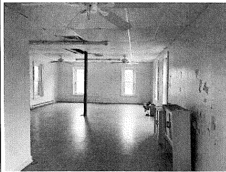
2 nd Floor Area - Peeling Paint
